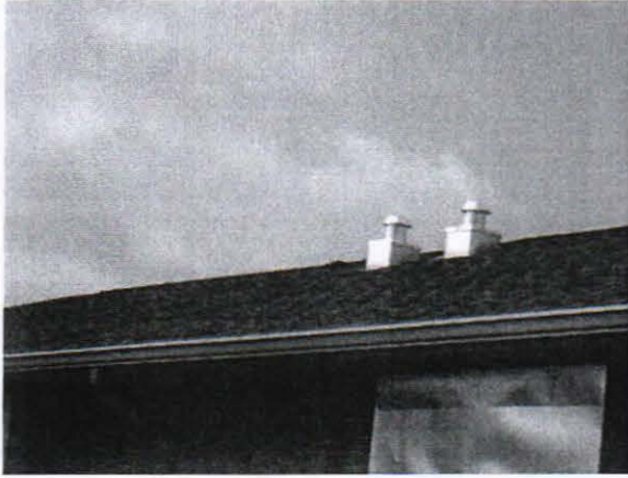
Mismatched Roof Caps
