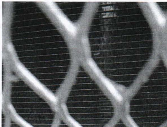
Condenser Coil Required Combing
