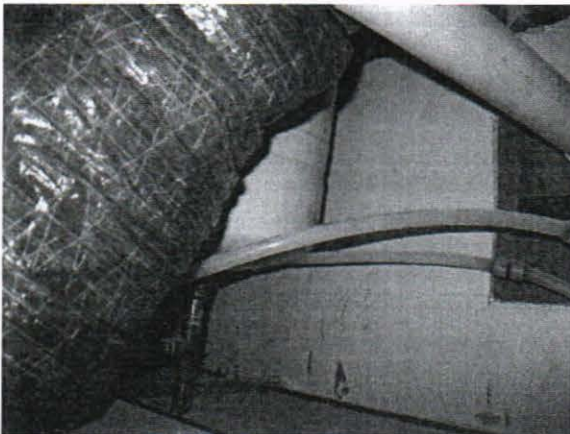
Water Pipe Missing Insulation
