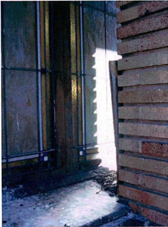
View from Southwest – Showing Wood Filler above Transom at North Side of West Masonry Pier
