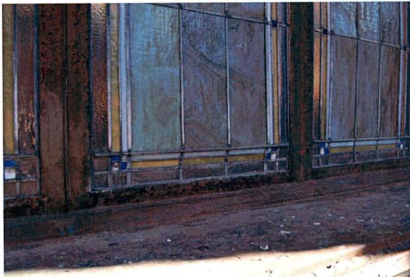
Deformed Area at Bottom of Art Glass Panel
