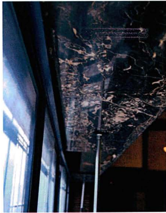
View of Underside of Transom, looking West, toward missing Soffit piece.
