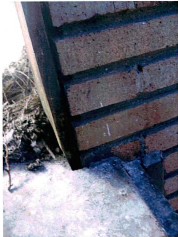
View from West – Showing Wood Filler and Gap Between Transom and North Face of West Masonry Pier
