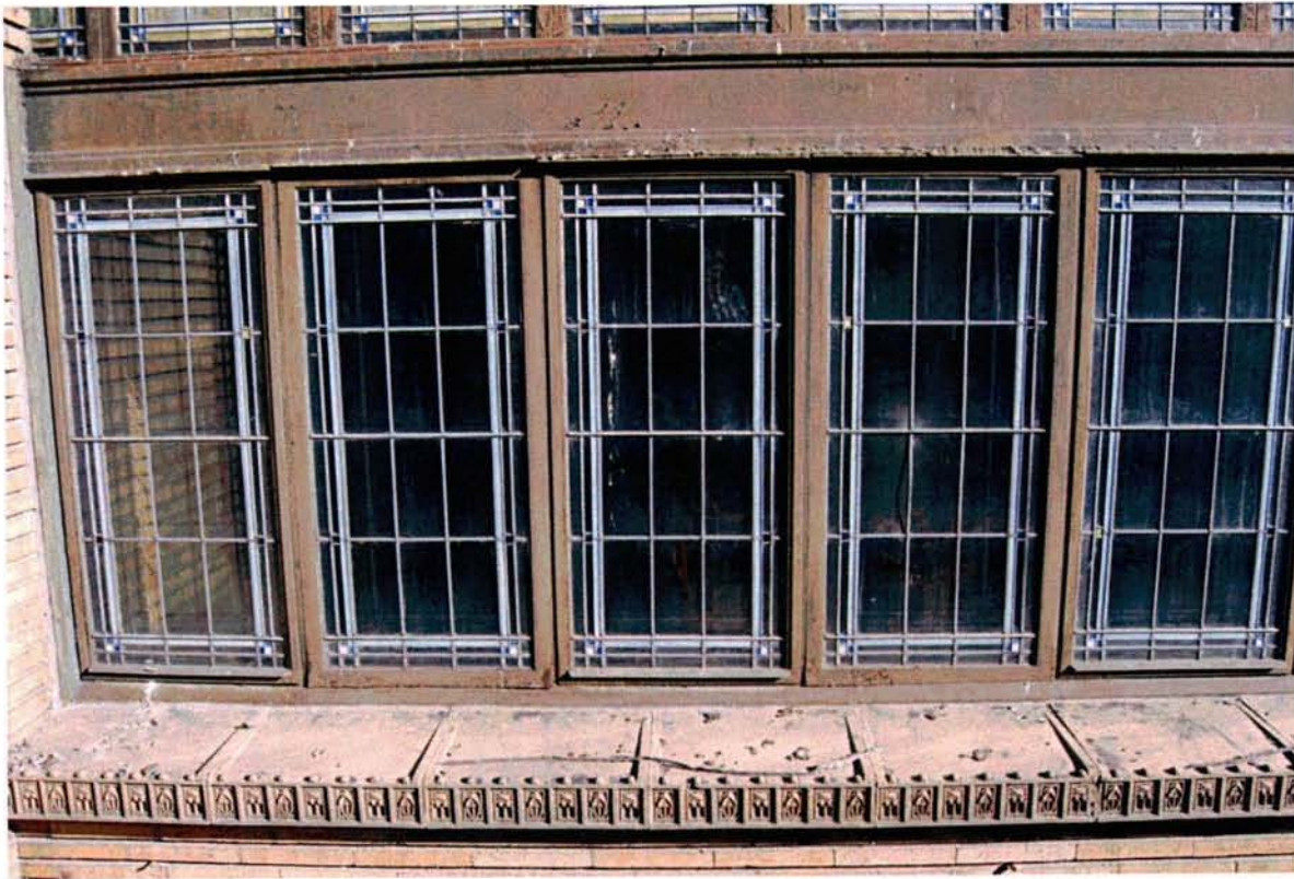
View of Fixed & Operating Sash - Note the deteriorated portions of the Fixed Window Sills
