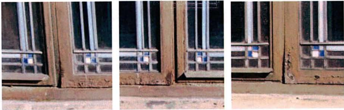
Closeup Views of Fixed & Operating Sash - Note the deteriorated portions of the Fixed Window Sills
