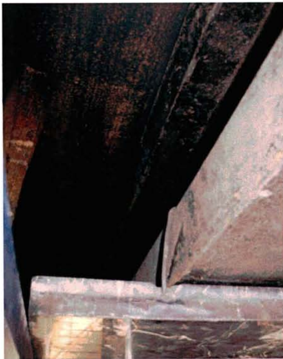
View of Underside of Transom, looking at Marble Soffit west of missing Soffit piece ; showing wire tie from connection to Marble Soffit vertically to where it clips over the steel support channel, above.
