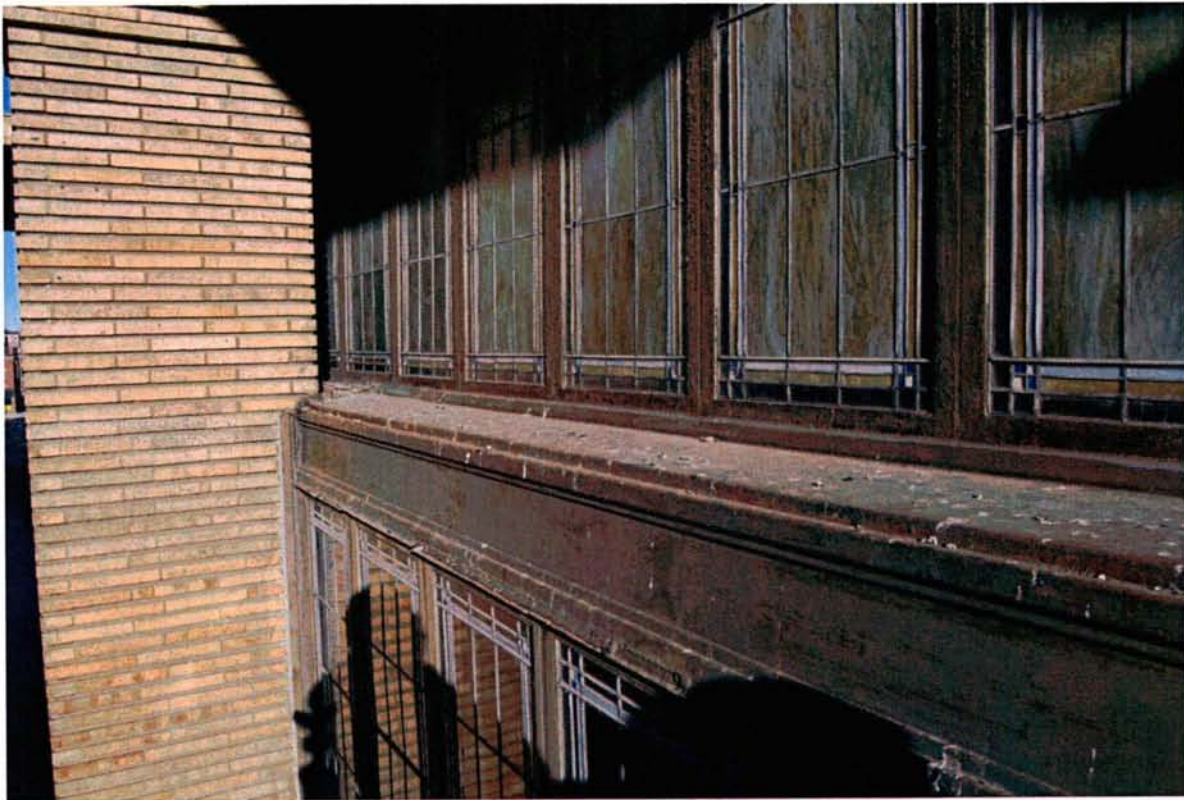
View along top of Steel Transom – Looking West (Note bird droppings and various areas of surface rust)
