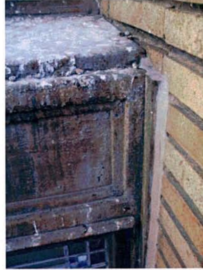
Top of Steel Channel at Steel Transom – East End of Lower Window Assembly - Filled with Sealant
