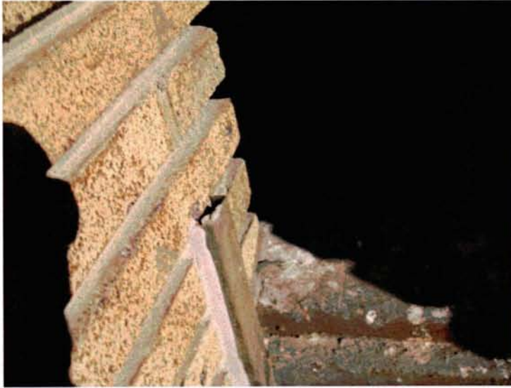
Top of Steel Channel above Steel Transom – East Side of East Masonry Pier – Sealant Missing
