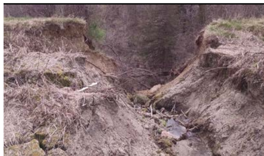
Oak Ridge – Breach of structure
