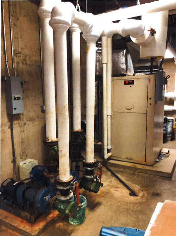
Figure 3.2: GHEX Circulation Pumps and Ventilation Heat Pump
