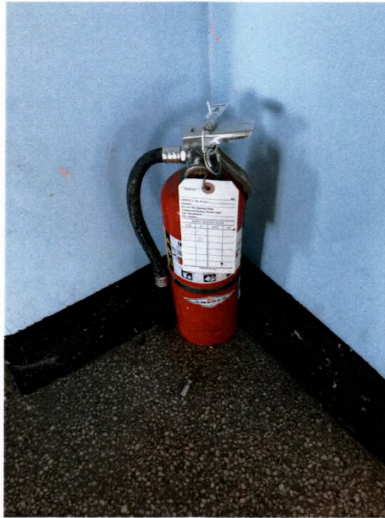
Photograph 13: Portable fire extinguisher, typical.
