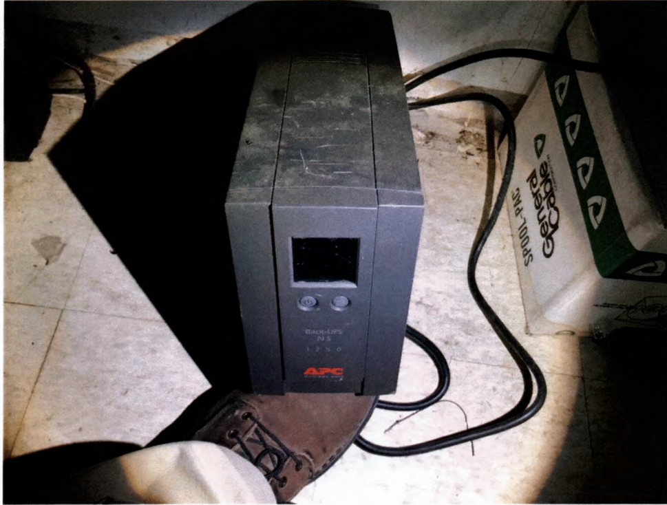
Photograph 5: Batteries (interruptible power supply)
