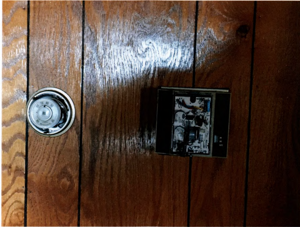
Photograph 15: Mercury-containing devices (thermostat), multiple variations.
