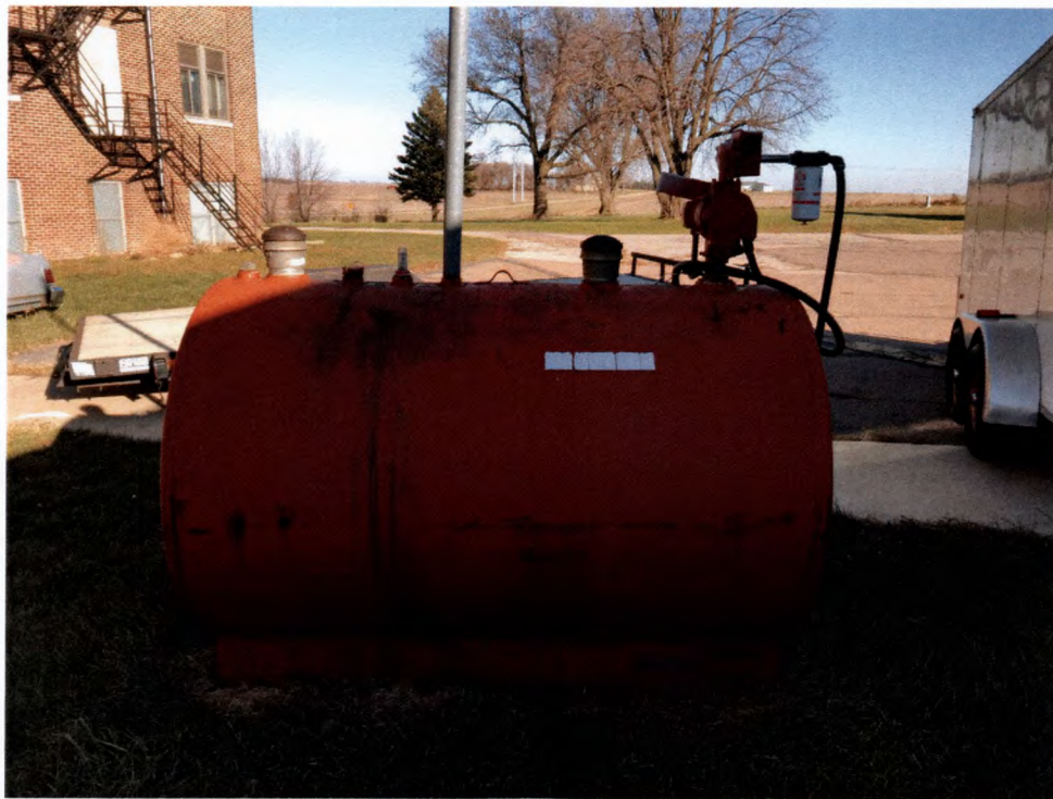
Photograph 20: Diesel fuel AST
