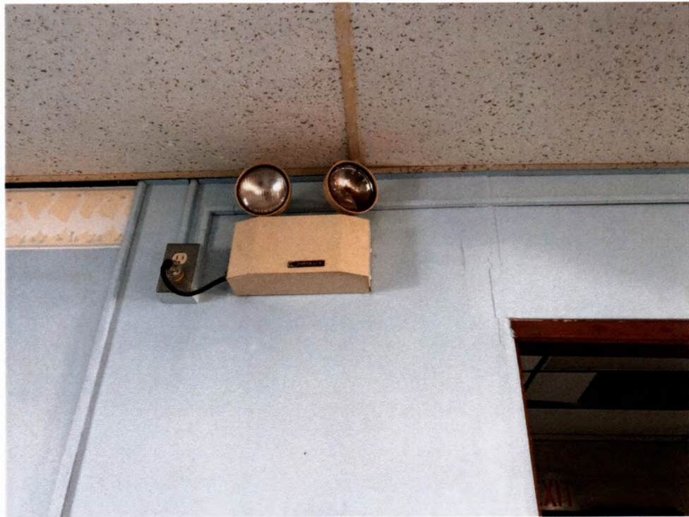
Photograph 10: Emergency lighting, typical
