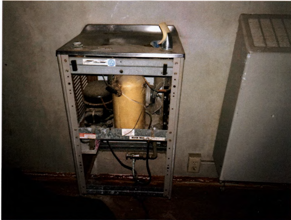
Photograph 7: CFC containing unit (water fountain)
