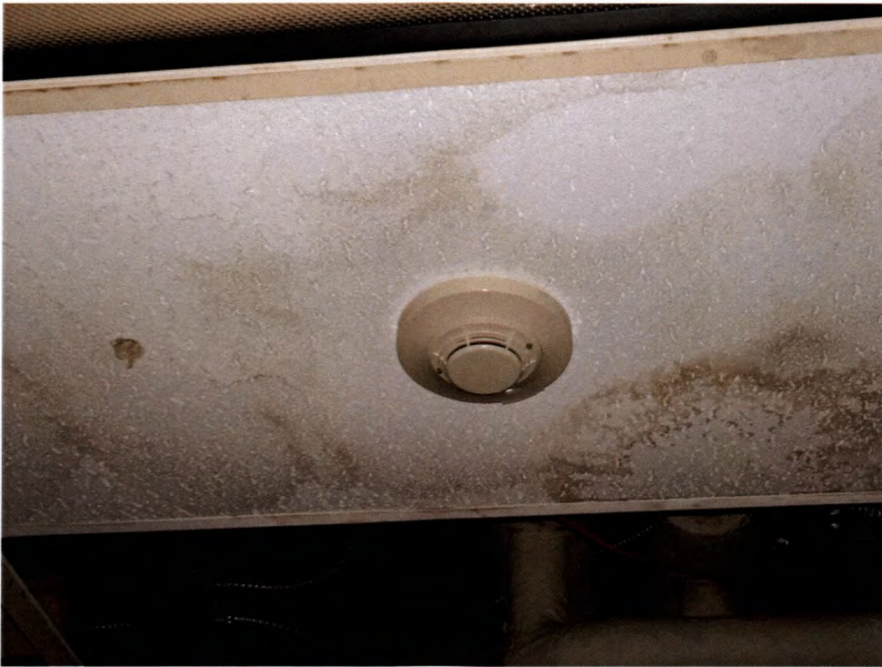
Photograph 18: Smoke detector, typical
