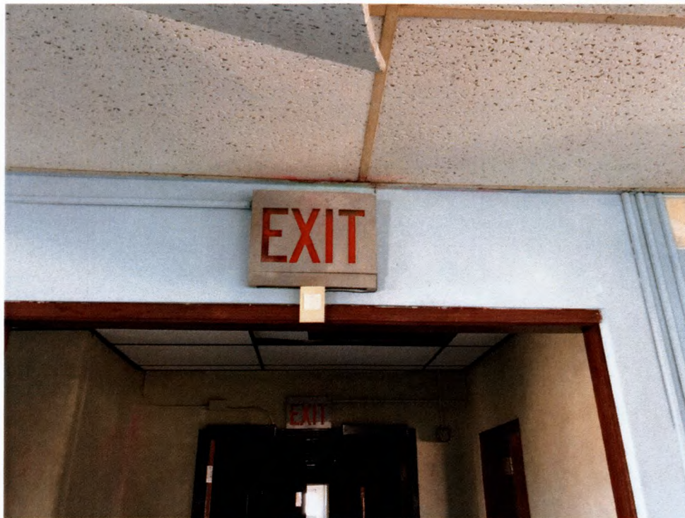
Photograph 12: Exit sign, typical
