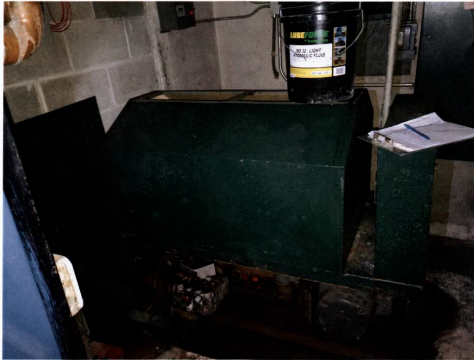
Photograph 11: Elevator, hydraulic pump
