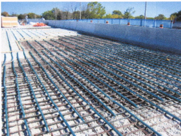
Galvanic anode system on bridge deck prior placement of reinforced concrete overlay
