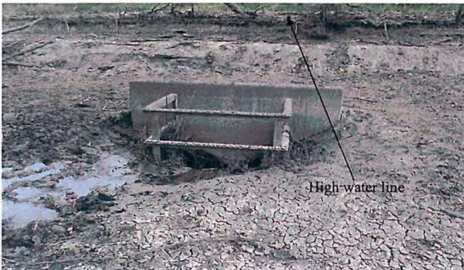
Normal flow 2 weeks later , notice how high water level was. Functioned as designed
