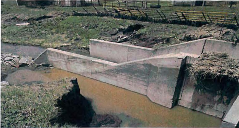
Eroded soils from concrete full -flow
