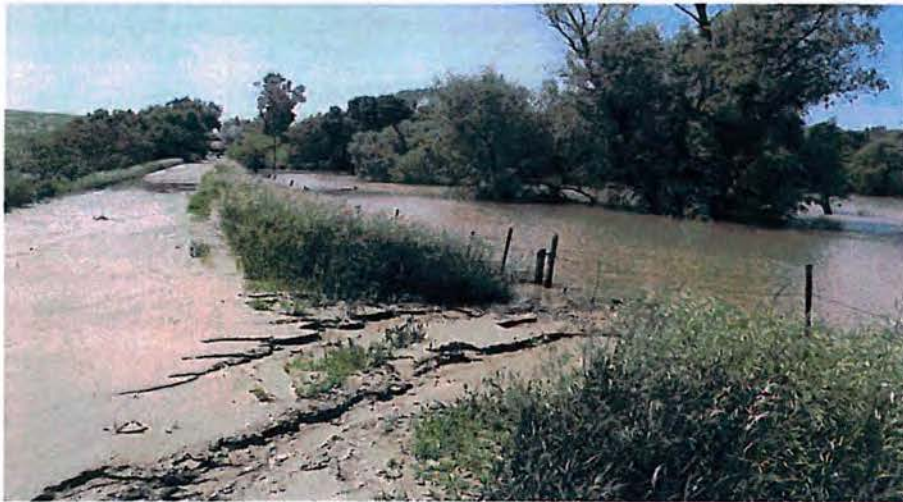
County dirt road structure after major storm event
