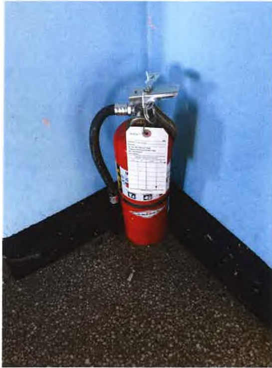
Photograph 13: Portable fire extinguisher, typical.
