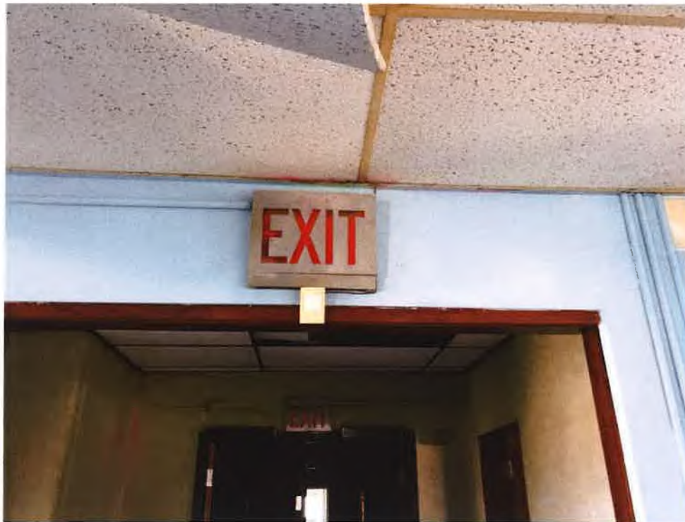
Photograph 12: Exit sign, typical
