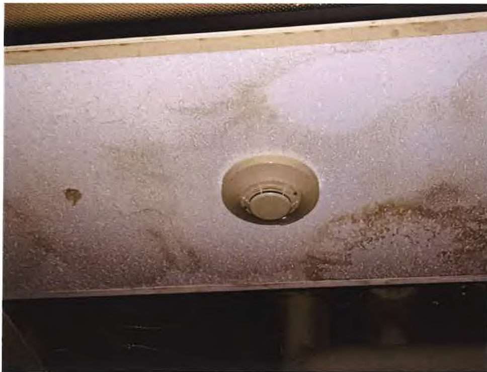
Photograph 18: Smoke detector, typical
