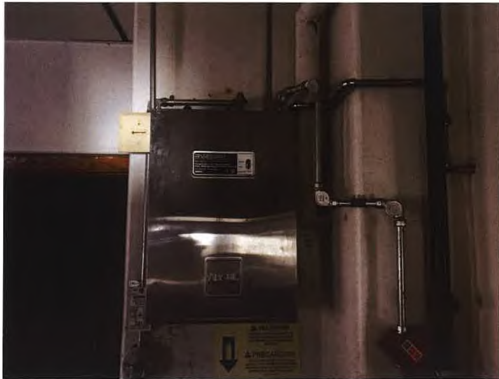
Photograph 14: Kitchen fire suppression system
