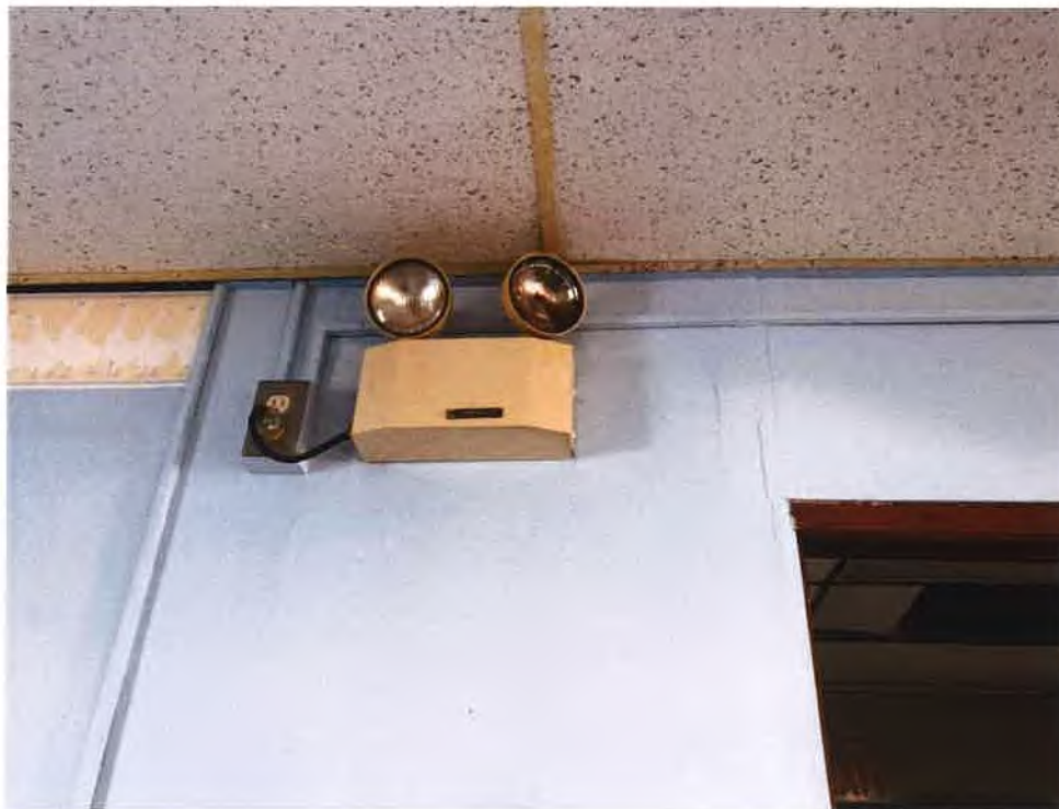
Photograph 10: Emergency lighting, typical
