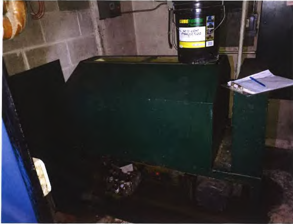
Photograph 11: Elevator, hydraulic pump
