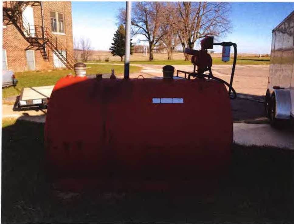
Photograph 20: Diesel fuel AST
