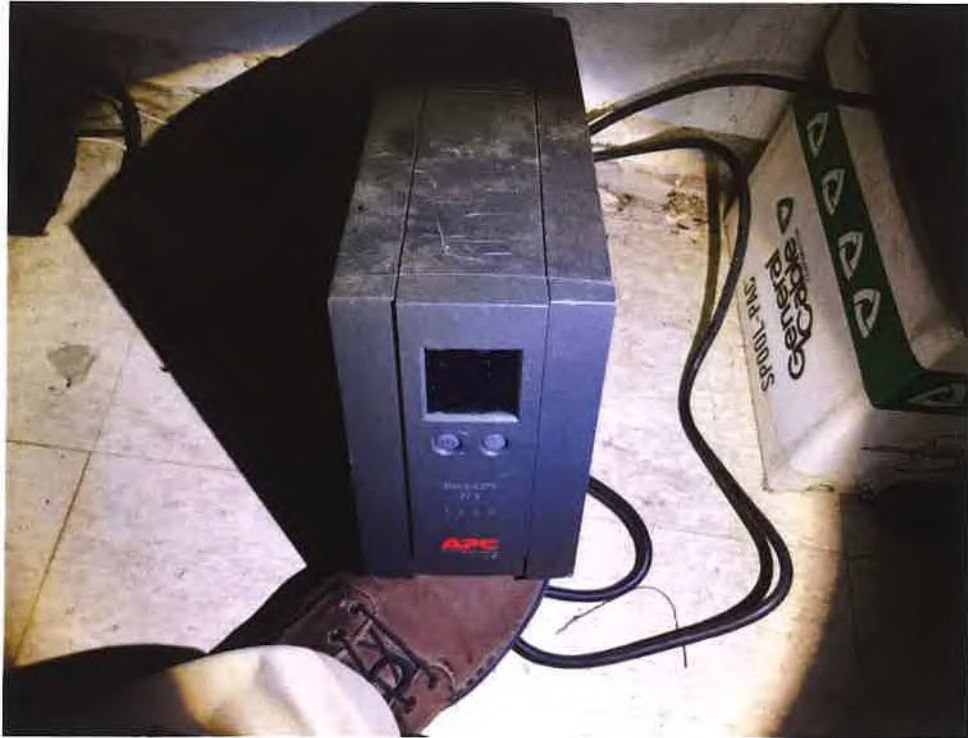
Photograph 5: Batteries (interruptible power supply)
