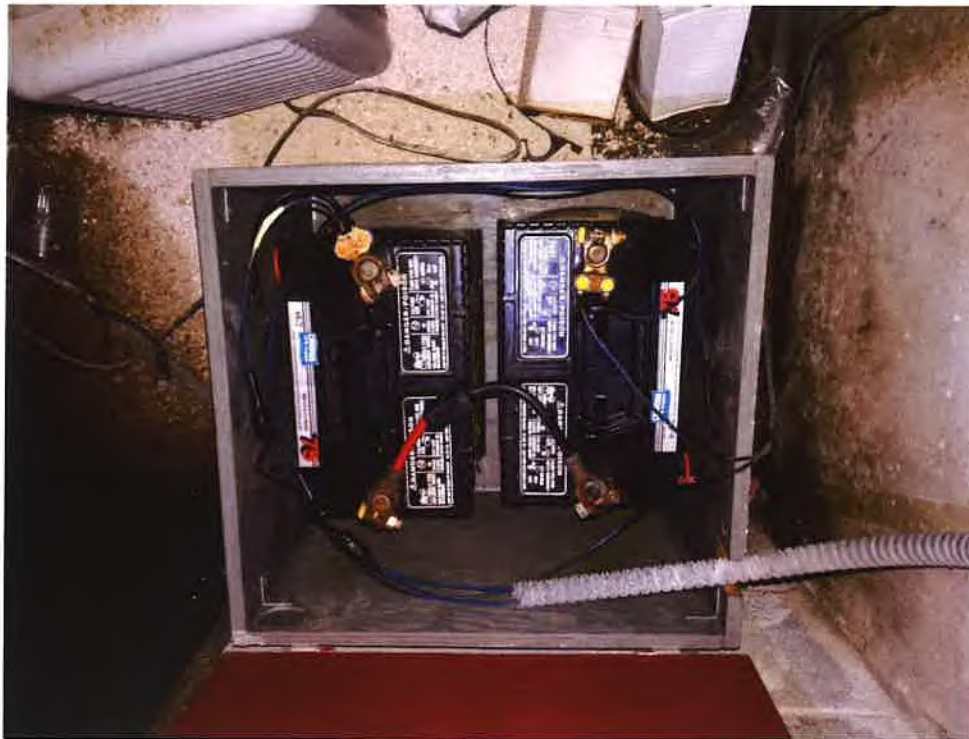
Photograph 4: Batteries (elevator backup power supply)
