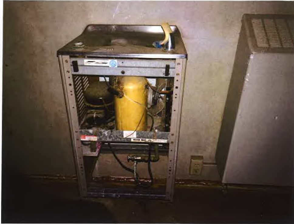
Photograph 7: CFC containing unit (water fountain)
