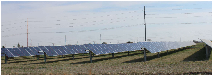
When solar projects reach the end of their expected performance period, there are several management options. They include extending the performance period through reuse, refurbishment, or repowering of the facility or fully discontinuing operations and decommissioning the project. | Photo by Rhea Landholm
