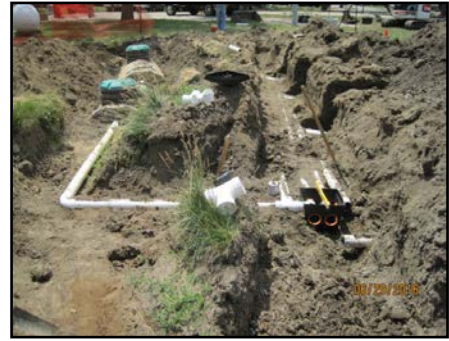
Brown's Lake – Septic System
