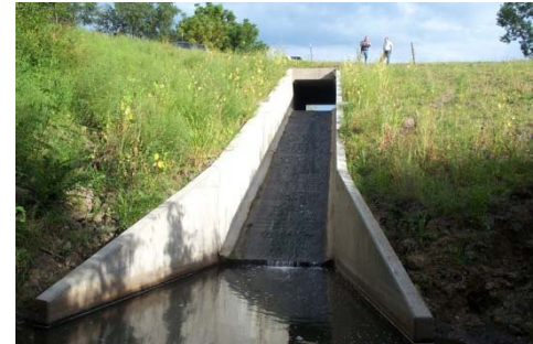
Top: 4 foot high sheet pile weir with a 1:20 grouted riprap slope in Crawford County. Bottom: RCB flume with 25 feet of fall in Fremont County.
