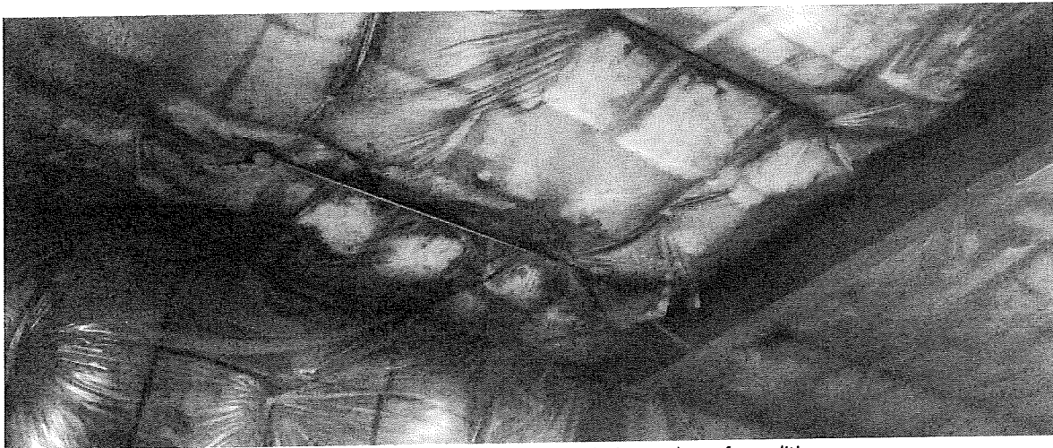
Ongoing roof leaks and deteriorated insulation contribute to structural decline and unsafe conditions.
